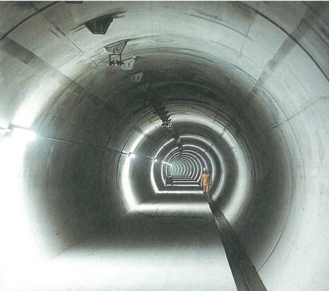
LEP tunnel before installation of bending magnets
